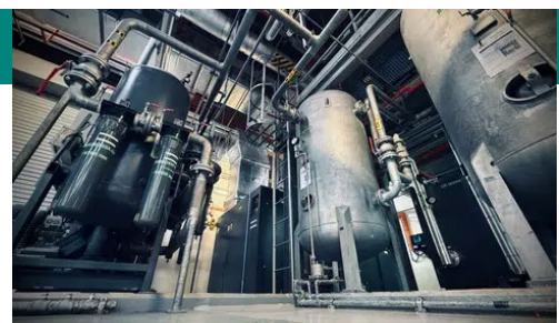
MSD's compressed air system
